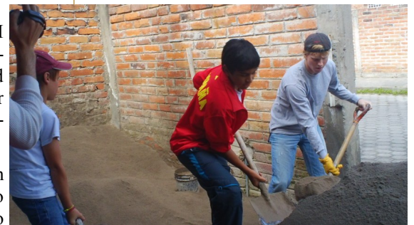
Anthony, Eduardo & Landon working on the sealing of the Ibarra, Ecuador church building.
